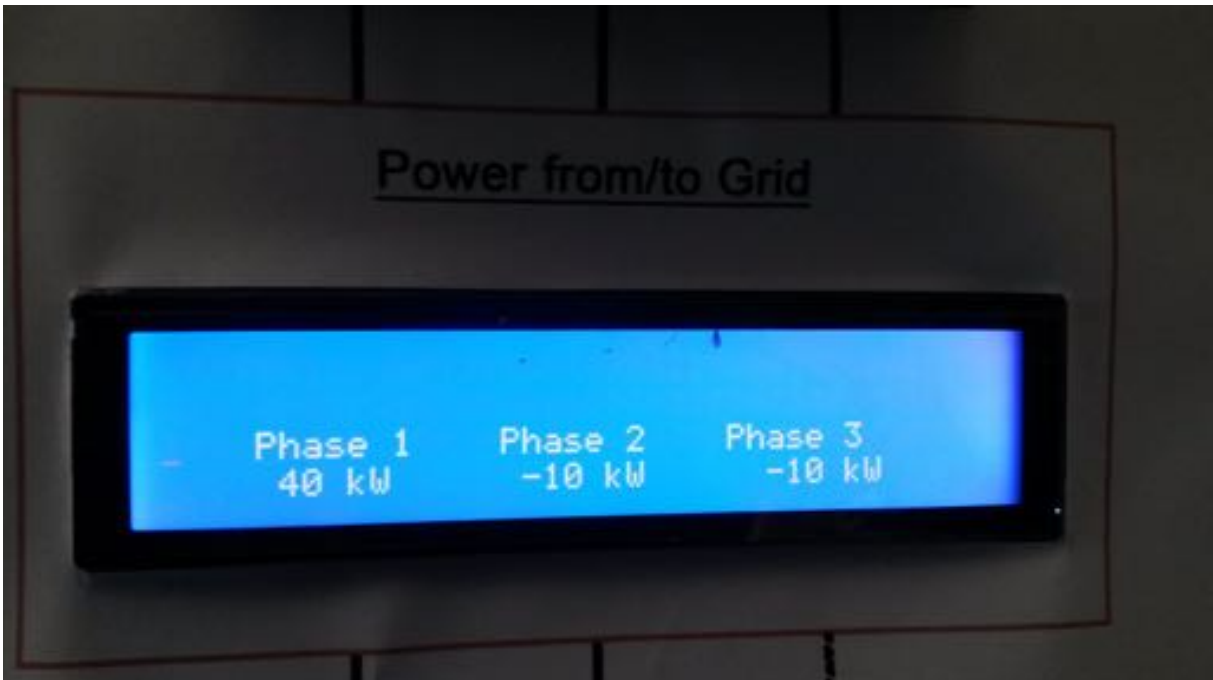
Figure 36, Grid information in substation platform
