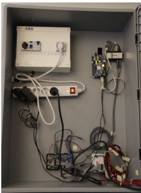
Figure 24, internal hardware setup
