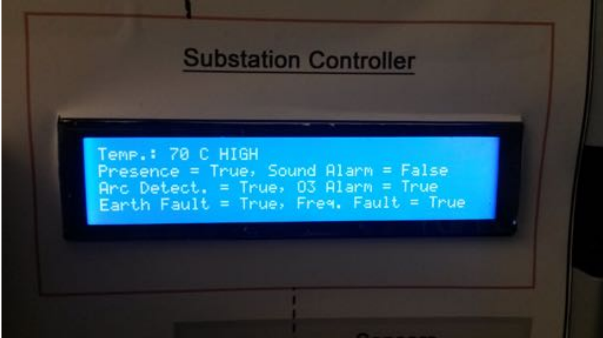
Figure 45, State of substation controller
