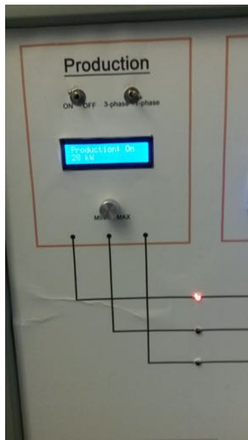
Figure 30, Production section of facility platform. State = On. 28 kW single phase
